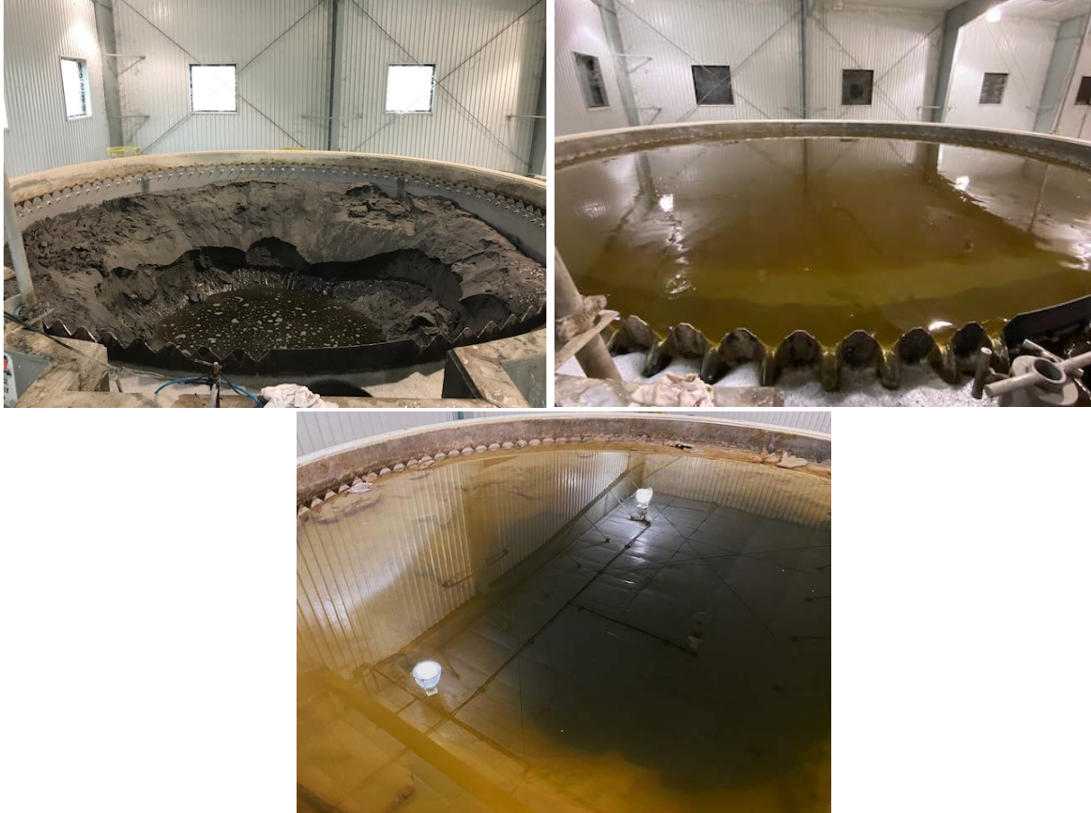
Figure 59: Pilot Reactor Clarifier Beaching
