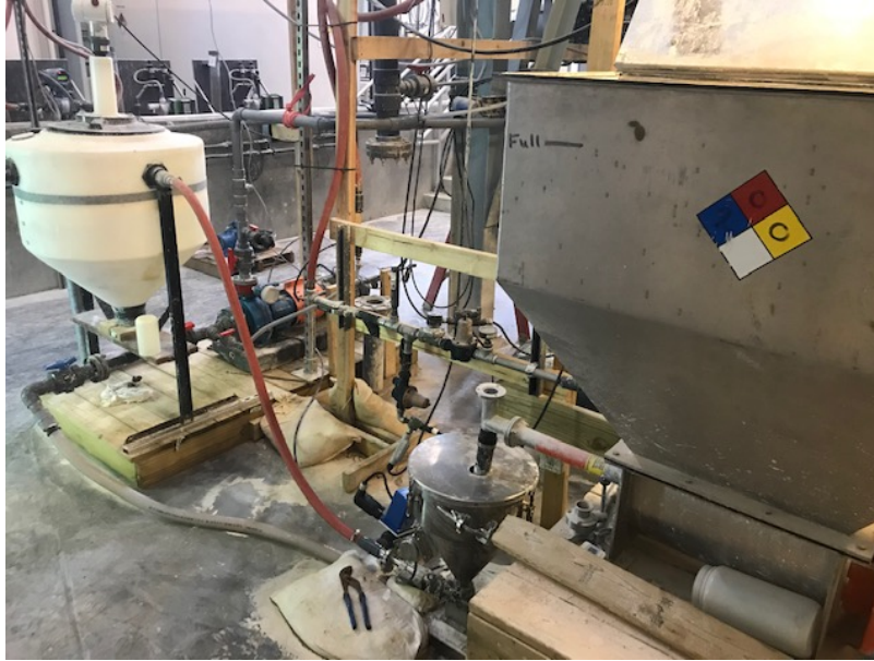
Figure 12: Automated Batching Configuration containing (from right to left) an MgO dry hopper, eductor cone, and recirculation loop for intermittent MgO slurry dosing
