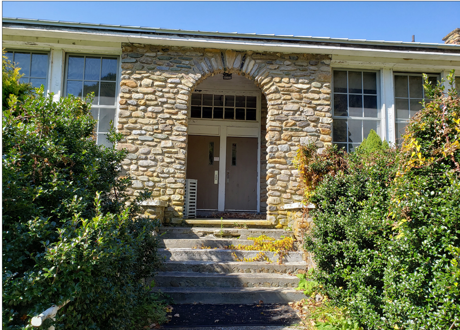
The stone schoolhouse entrance is in good shape, but only accessible by stairs without hand railings. The plants on either side of the entrance are overgrown.
