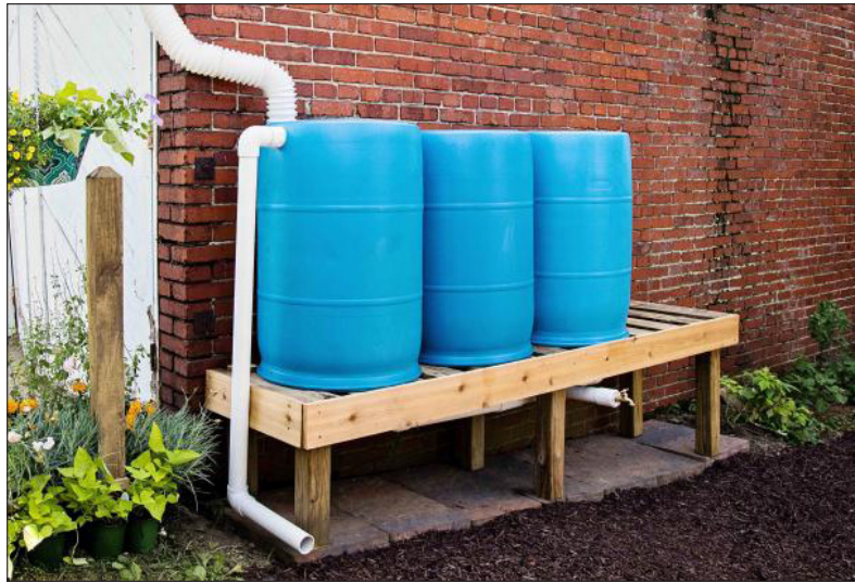
Rain barrels in a system such as this provide additional capacity to manage rainwater runoff from the building and give children a chance to learn about hydrology.
