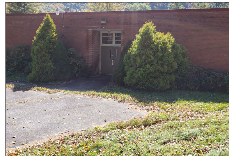
An entrance to the brick addition. The 1950s-era addition is in poor condition with several known water leaks. The County plans to remove this portion of the building.
