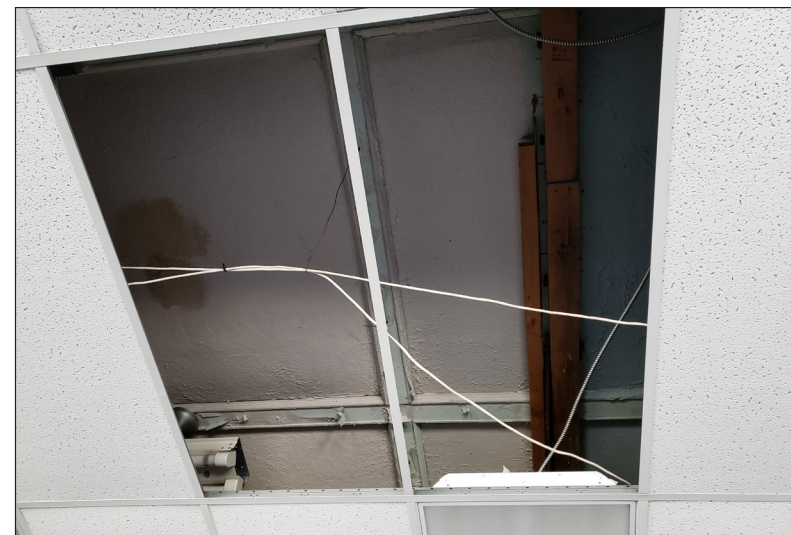
A view through the ceiling panels of the dropped ceiling to the original. Height of original is 11'8" and there is an opportunity to expose them.
