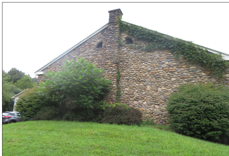
A view of the roof line and chimney details. The roof of the old stone school portion appears to be in good condition with no water damage visible on the inside.
