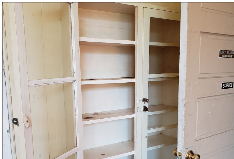
Original built-ins and shelving in the classroom to the left (when entering the front door). Shelving is in good condition.
