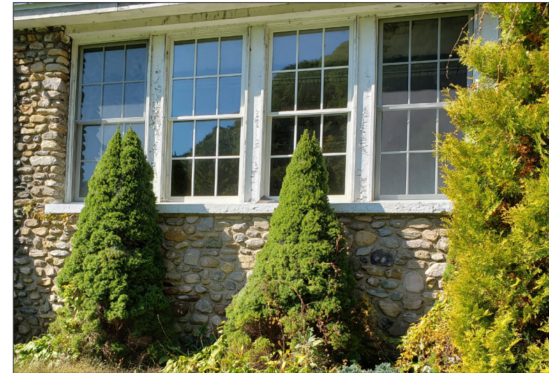
The windows appear to be in good condition with the exception of some chipping paint and need for general cleaning.
