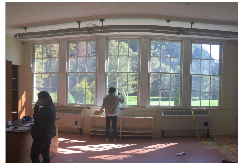
Large windows are in great condition and found in all classrooms/rooms. The windows provide lots of natural light and views to the scenic landscape outside.
