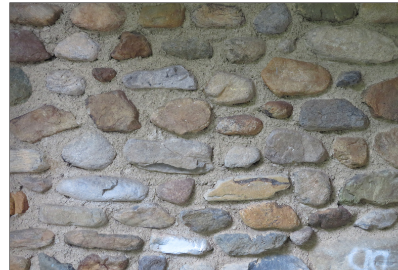
The original stone and mortar joints of the building appear to be both in great condition.
