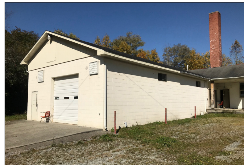
The storage building is located behind the original rock school. It is in better condition than the main brick building and has the potential to be included in the redevelopment planning process.
