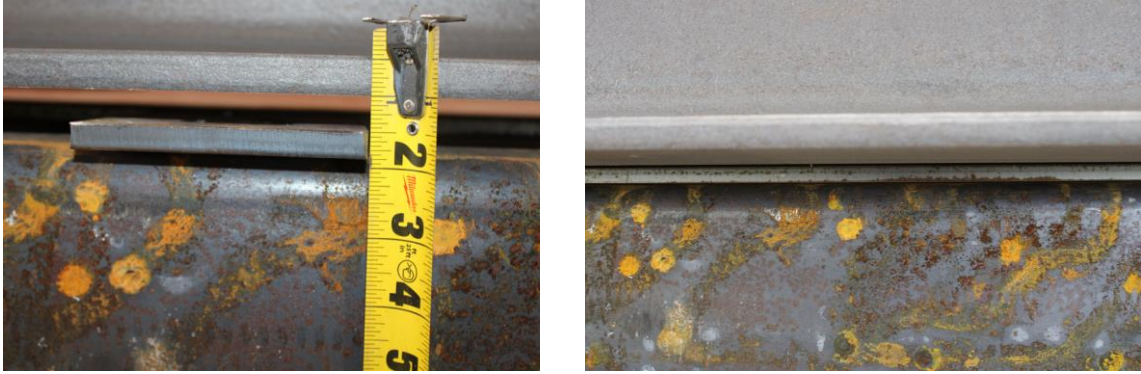
Figure 6-7. Gap between plate and beams before and after the use of the hydraulic pump
