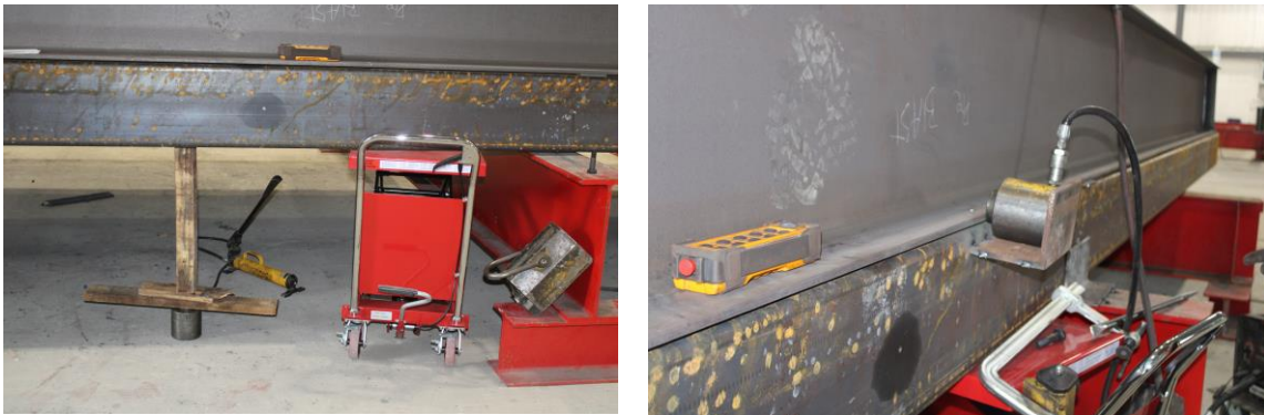
Figure 6-8. Use of hydraulic press to reduce the gap between the plate and beams
