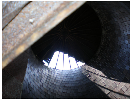
Figure 4-7: Silo roof damage
