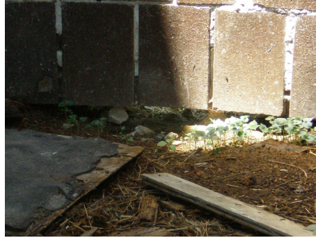
Figure 4-5: Earthen floor and foundation gaps
