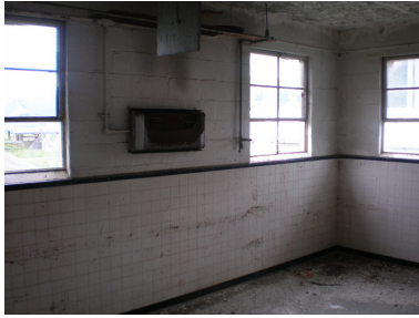
Figure 4-11: Bottling room plumbing
