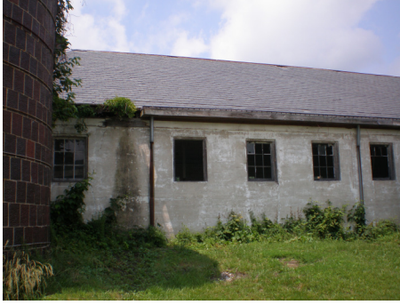
Figure 4-8: Missing and broken windows
