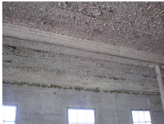
Figure 4-10: Peeling lead paint
