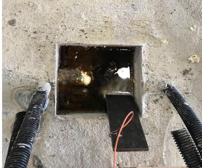
Figure 3-10 The Block Out During the Corrosion Experiment
