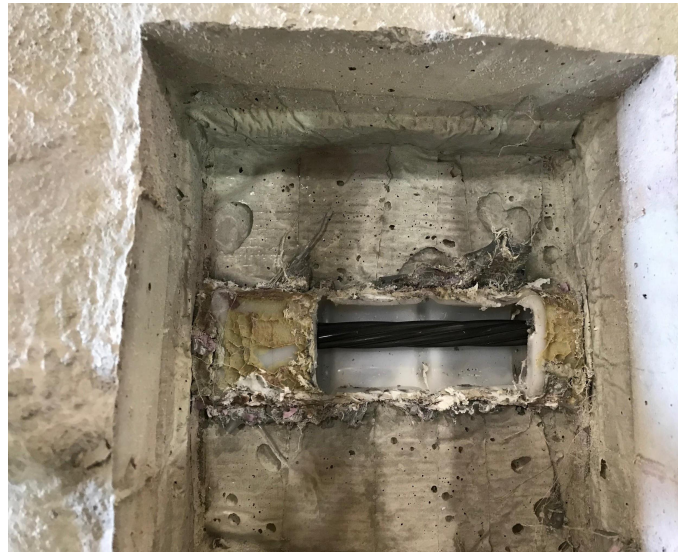
Figure 3-7 A View of the Block Out After the Duct was Cut Off
