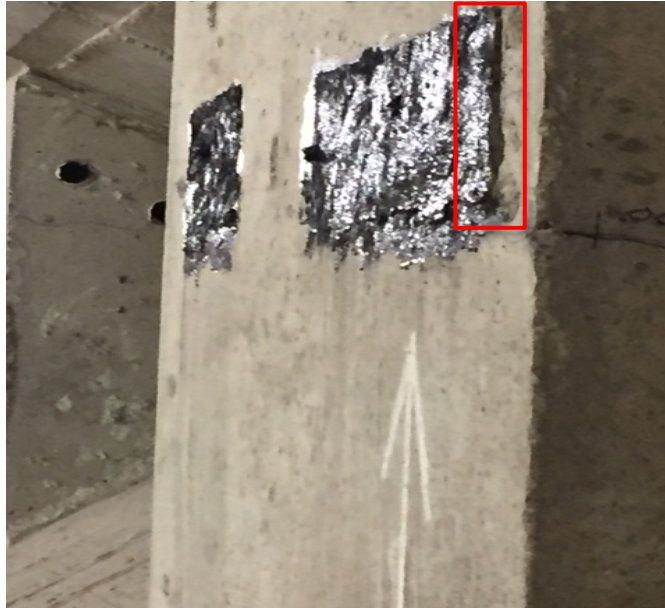
Figure 1-5 The Dislodged Block Out Pocket on the Inside of the Varina-Enon Bridge
