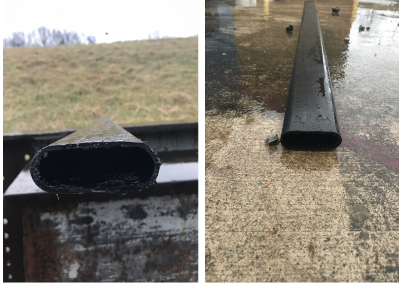
Figure 3-15 View of the Smooth Duct
