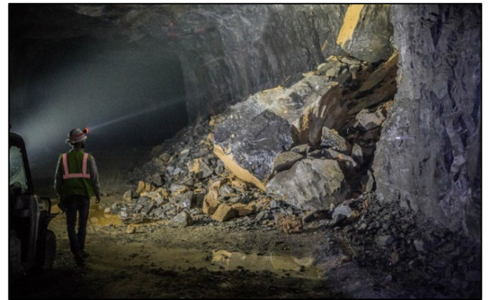
Fig. 2. Ground collapse from karst cavity in the case study mine pillar (Bishop, 2020).
