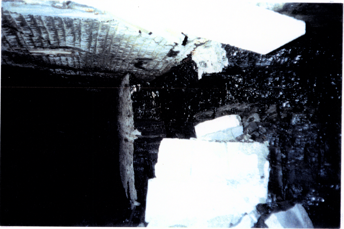
6.4 Photograph showing excessive rib spalling
