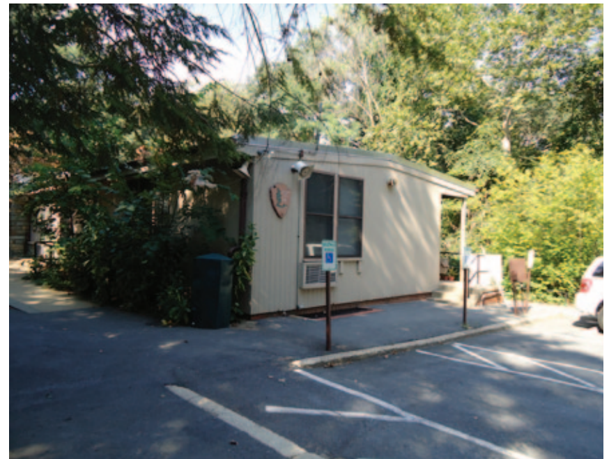
Portion of existing building closest to parking lot next to main entrance
