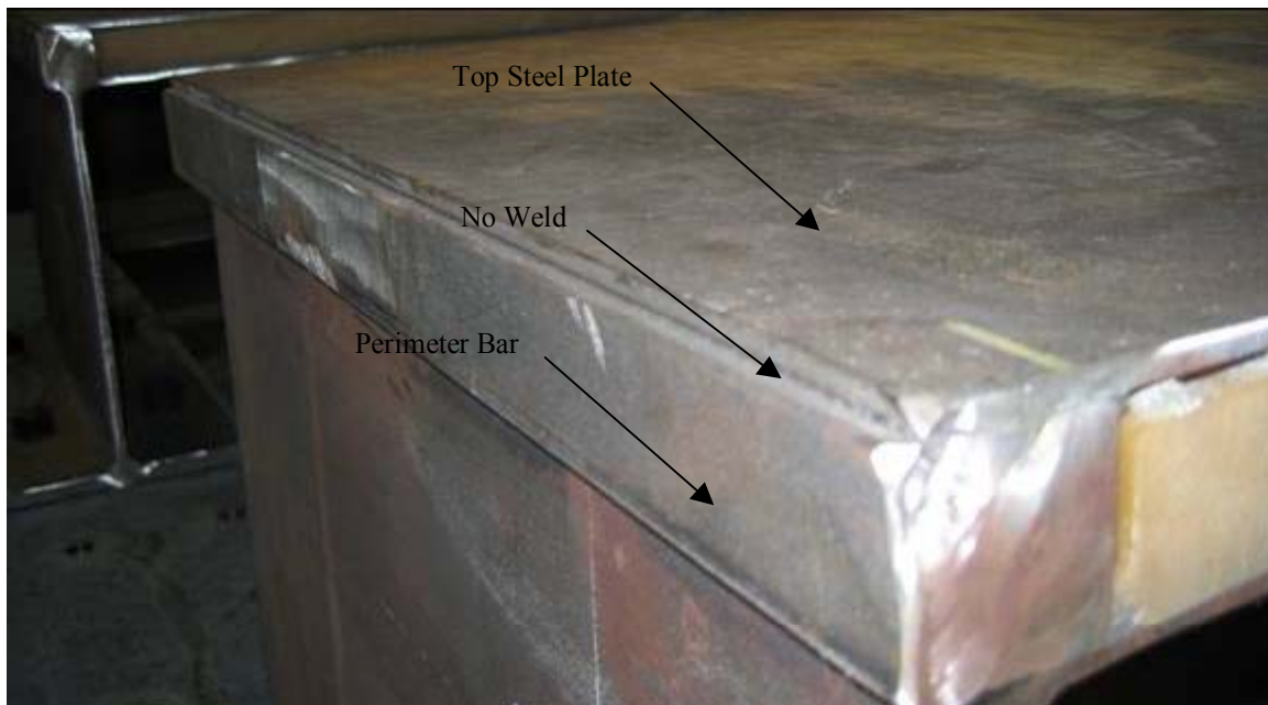
Figure 5.2 Top Steel Plate and perimeter bars not welded
