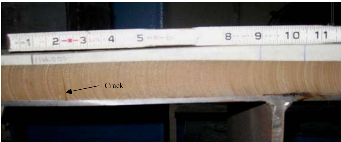
Figure 4.4 Cracked core of Panel 4 on the left cut edge
