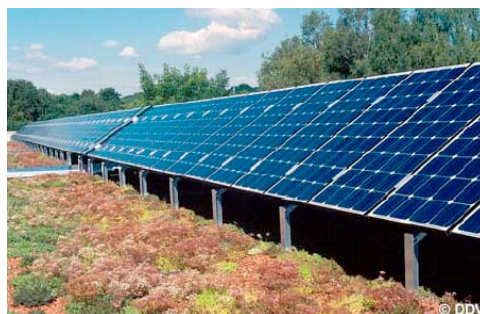
Figure 3.5 - Photovoltaic installation combined with extensive green roof on a school near Stuttgart (Appl & Ansel, 2004, p. 323), permission to use granted by: Jennifer Sprout, Green Roofs for Healthy Cities (Jan. 25, 2007)
