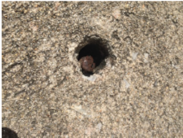
Exposed rebar in pavement & wall
