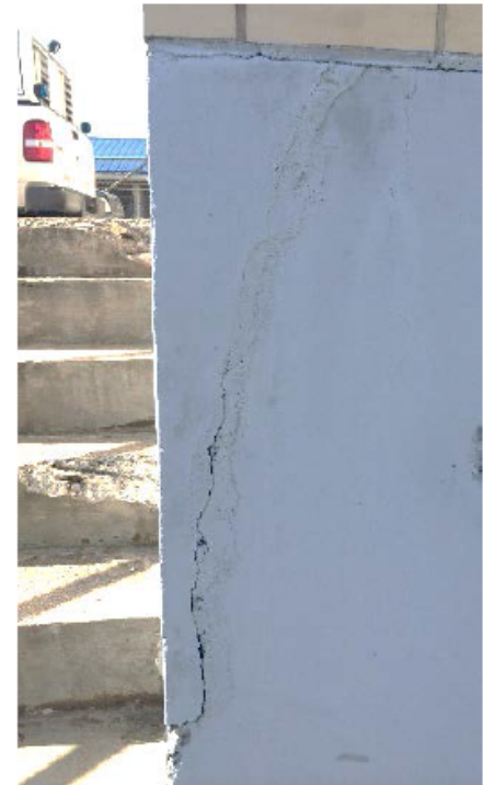
Cracks on concrete surface
