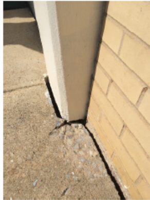
Gaps near foundation
