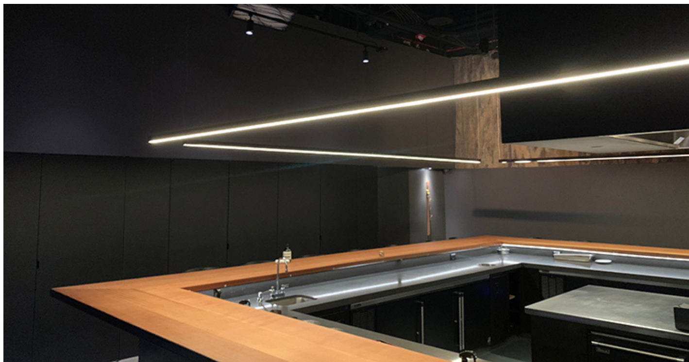
Gozu installed a hospital-grade system that safely sanitizes ceiling air in the intimate 45-seat restaurant.
