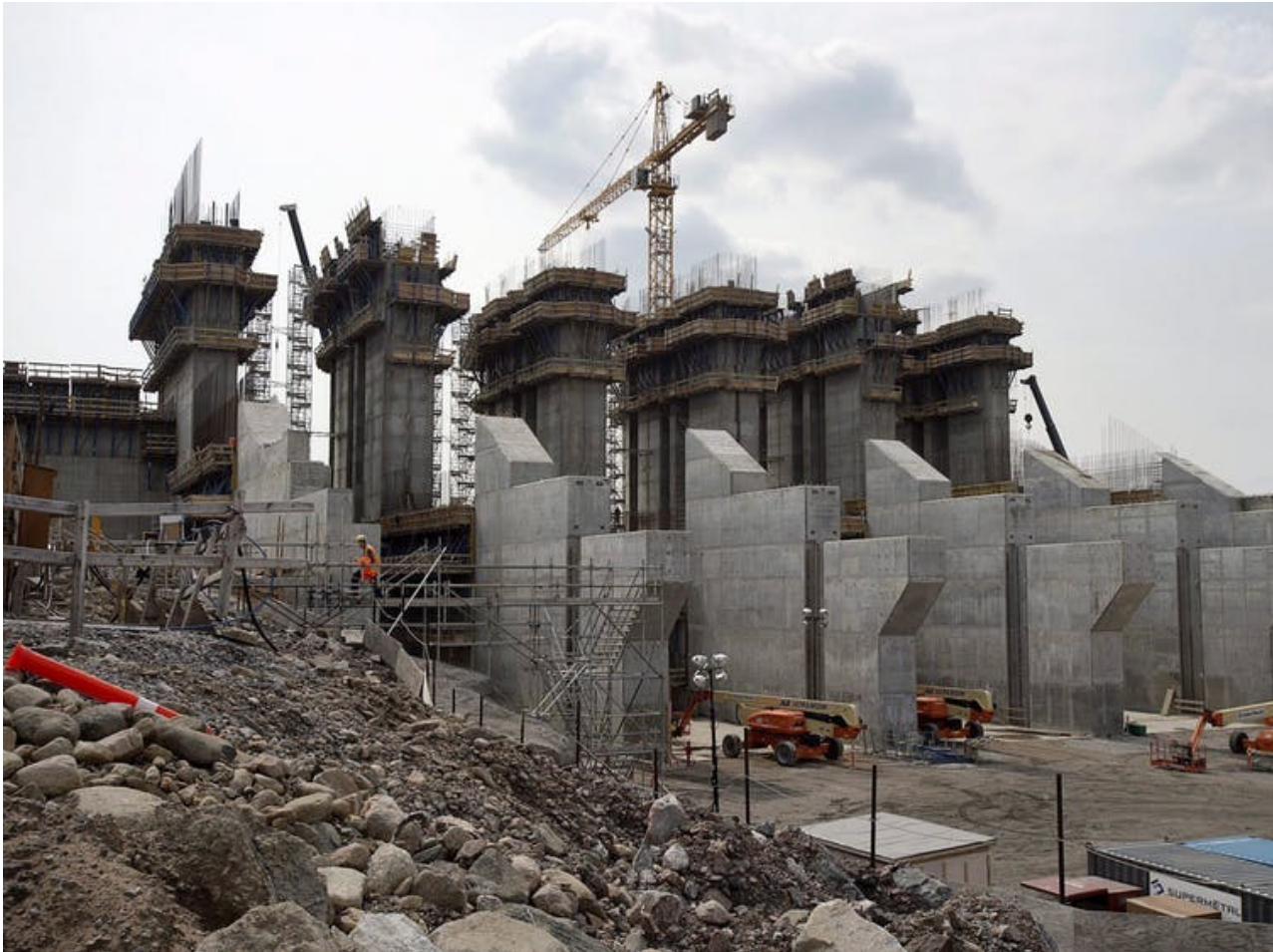
The construction site of the hydroelectric facility at Muskrat Falls, Newfoundland and Labrador is seen on July 14, 2015. THE CANADIAN PRESS/Andrew Vaughan
