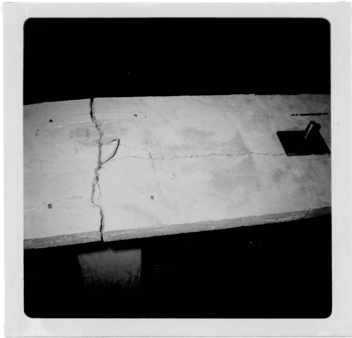
Figure 15. Support Crack Pattern on Top Surface
