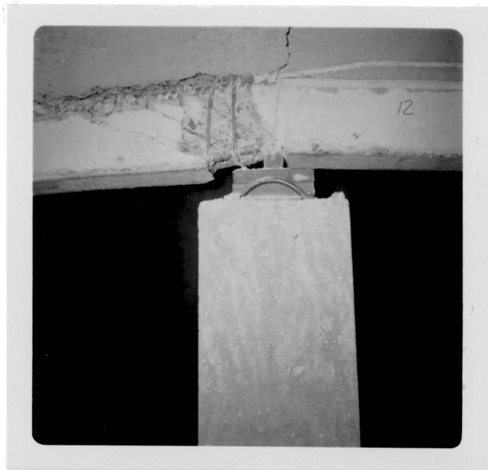
Figure 14. Appearance of Failed Support Section, Beam No. 3
