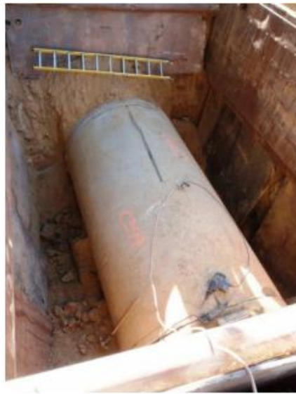
Figure 2-10: Example of Direct Assessment (Courtesy WSSC, 2025)
