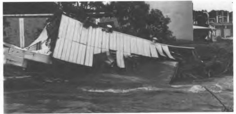
The building that was once the office and warehouse for a gas and oil firm withstood the 1979 flood but failed to withstand the Mayo River for a second time.
