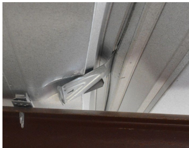
Figure B-32 Clip damage of Specimen 8
