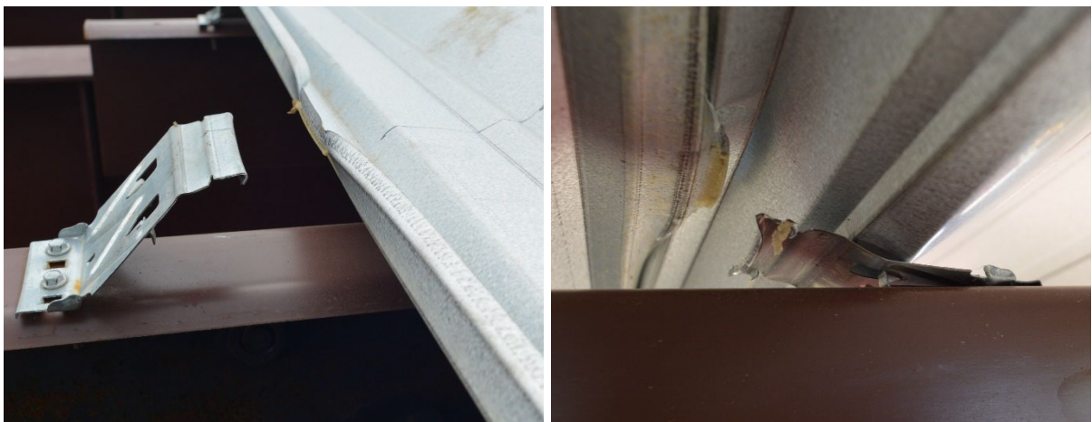
Figure B-44 Clip damage of Specimen 11
