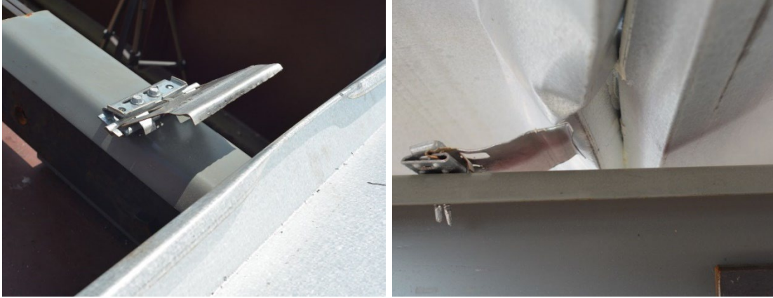
Figure B-24 Clip damage of Specimen 6
