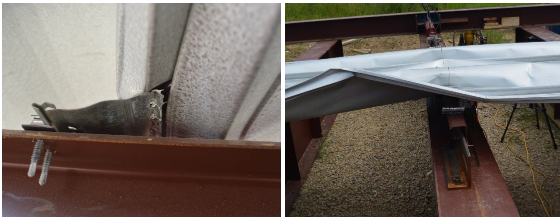
Figure B-20 Clip damage of Specimen 5
