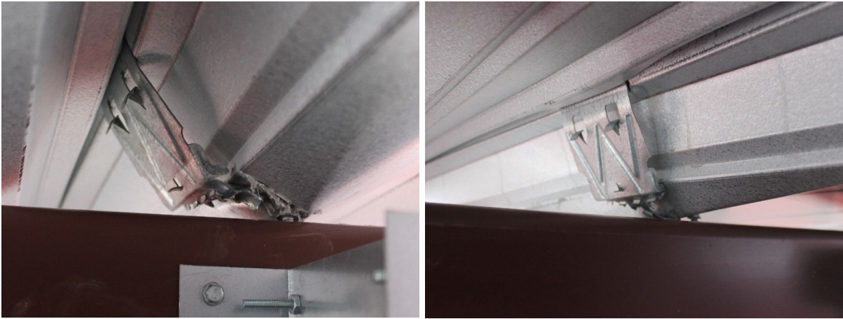
Figure B-28 Clip damage of Specimen 7
