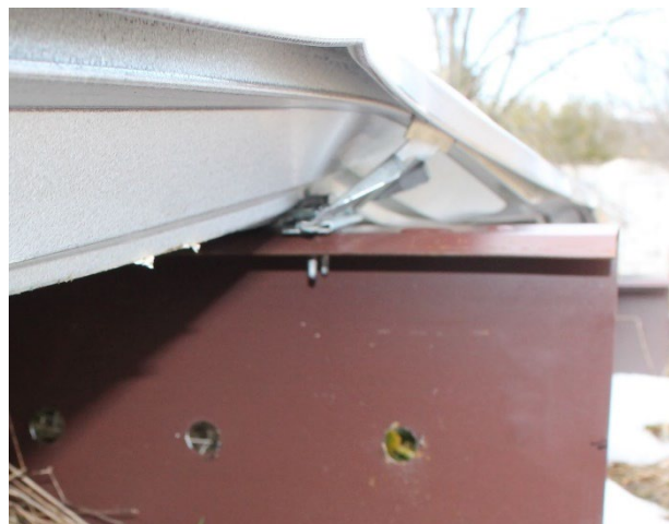
Figure B-8 Clip damage of Specimen 2
