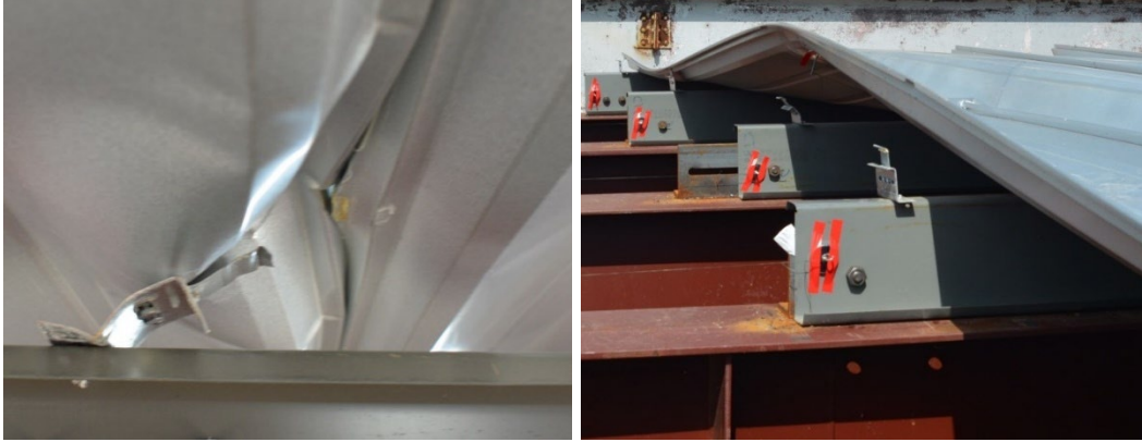
Figure B-12 Clip damage of Specimen 3
