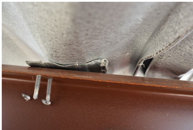
Figure B-16 Clip damage of Specimen 4
