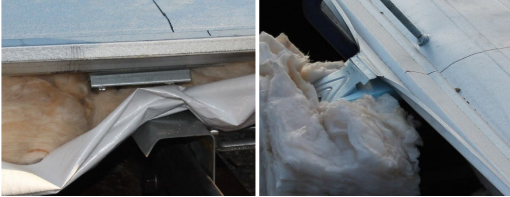
Figure B-36 Clip damage of Specimen 9
