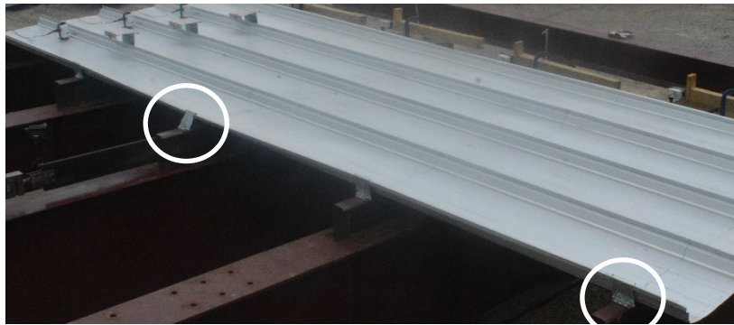
Figure 6-14 Typical deformed configuration with clip bending (from Specimen 7)
