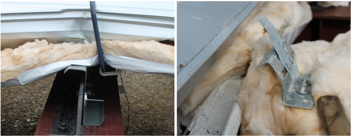
Figure B-40 Clip damage of Specimen 10
