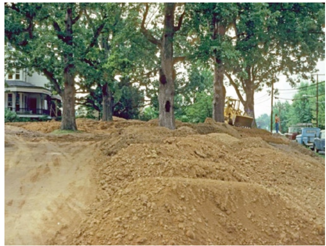
Figure 3.5. Inappropriate addition of topsoil over native trees: The topsoil material was added too thickly (12 inches) and then compacted (as seen at left) to a point that gas exchange by the living tree roots was limited. Most of these white oaks died within two years of this application.
