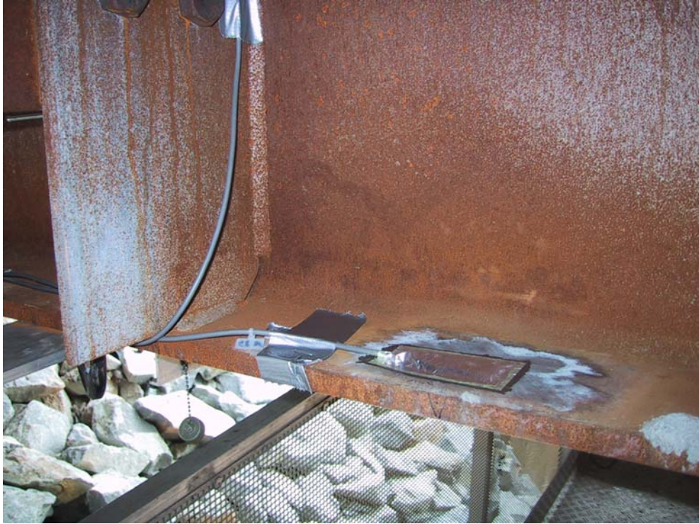
Figure 3.4: ER Strain Gauge on Steel Girder
