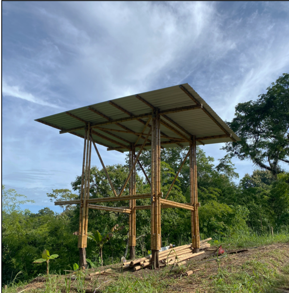
Figure B4. Finished Framing and Roof Installed. Triangular members in the walls and cross-bracing between the roof beams resist lateral forces. “Botas y sombrero”
