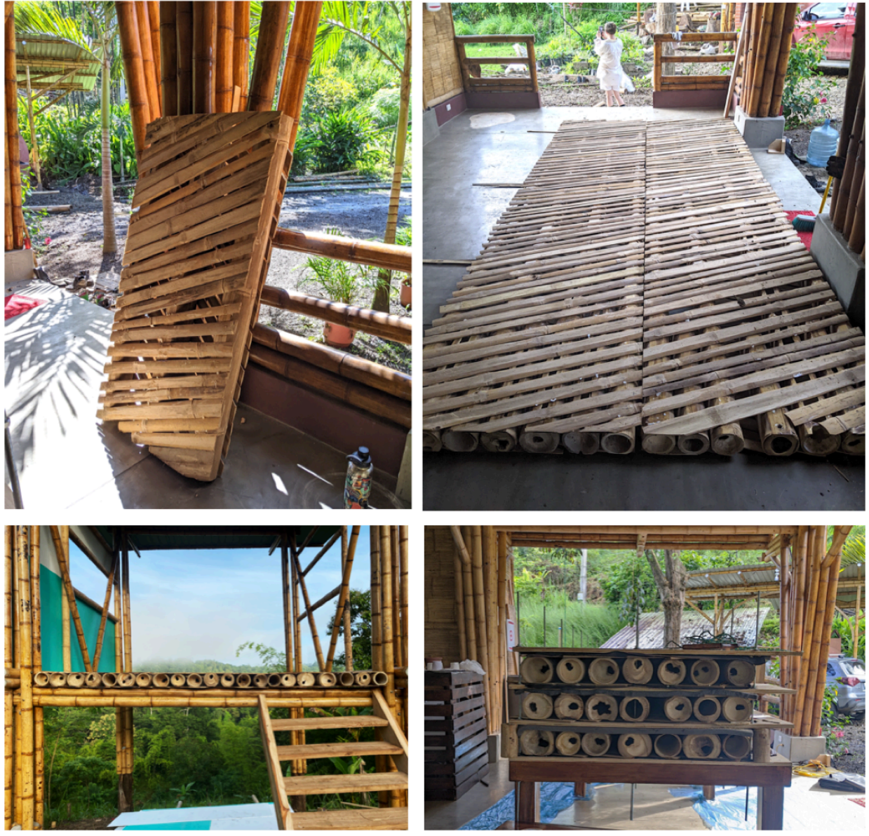
Figure 19. Panels. (top left) 2'x6' test panel. (top right) Full-scale 1m x 4.5m panels. (bottom left) All three panels installed in structure. (bottom right) Panels stacked on press mechanism.
