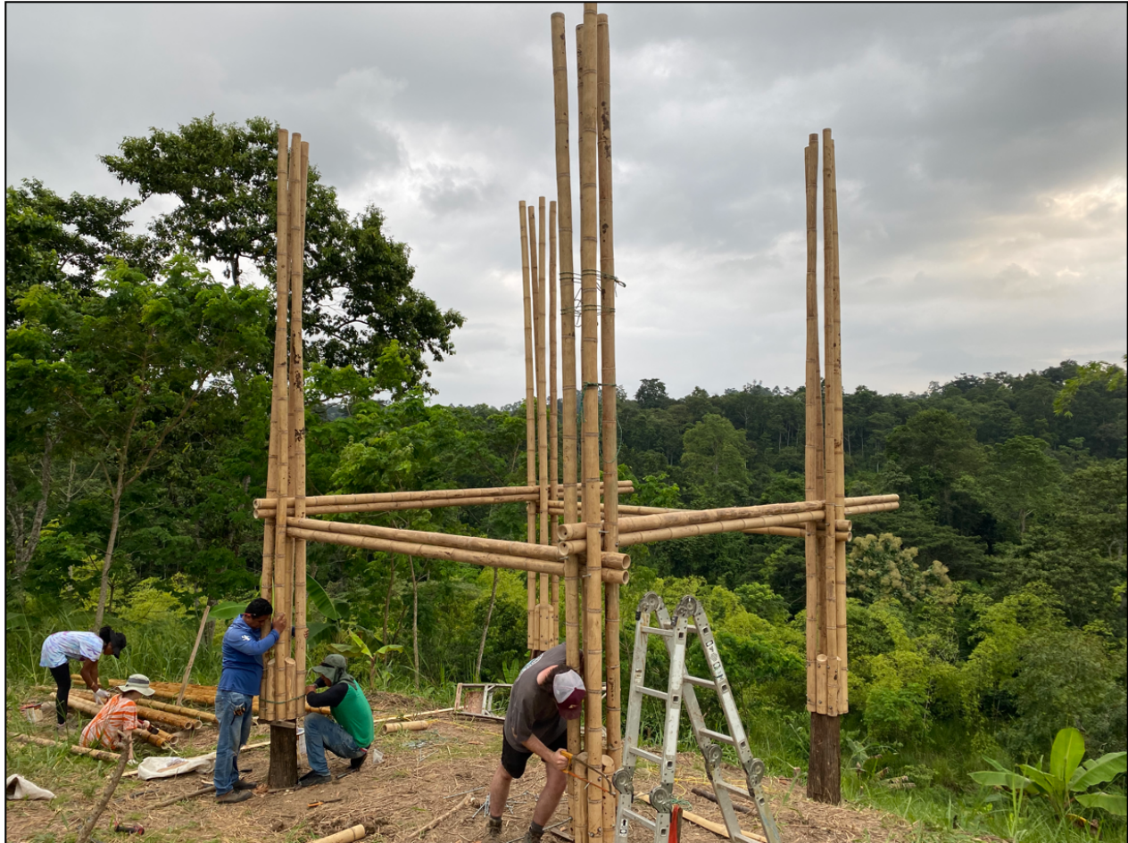
Figure B1. Early Framing Process. Local bamboo maestros utilize rope to temporary hold bamboo in proper positions. VT student cuts off extra threaded rod from foundation connection- threaded rod is initially cut longer than needed to ensure easier workability and then trimmed after installation.
