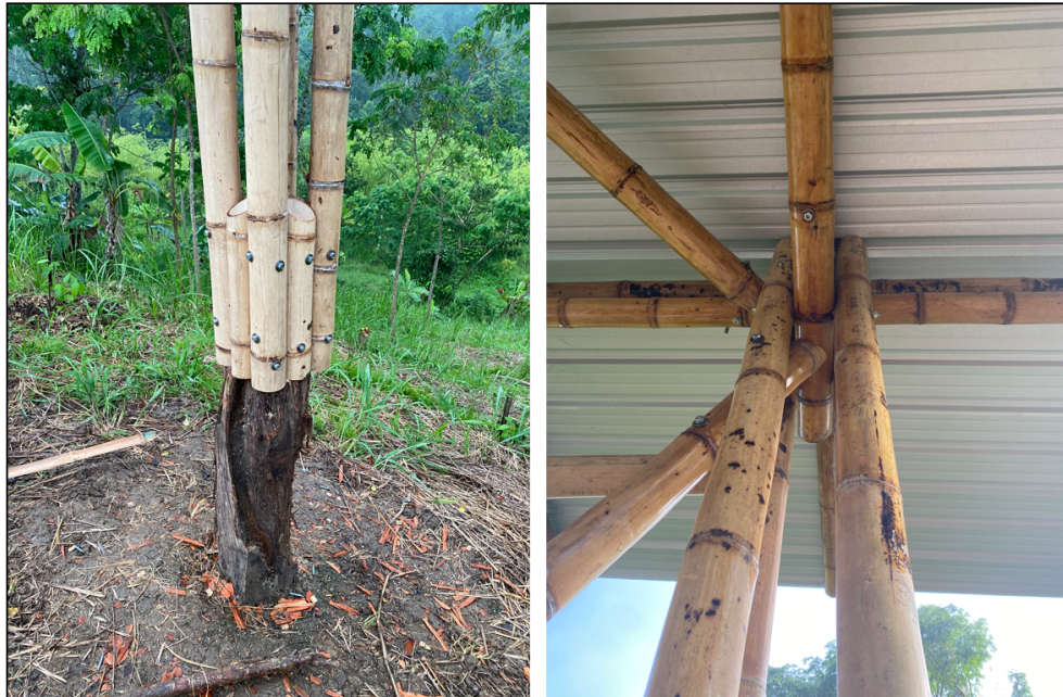
Figure B6. (left) Foundation connection. The group is connected to each other in two directions and then anchored to the teak stump. Notice the stark color difference between this bamboo and the varnished bamboo to the right. (right) Column to roof joint. While beautiful and interesting, this is a good example of how intricate traditional bamboo joints can be. A four-culm column, roof joist, roof cross-brace, and two wall members all meeting in one corner. The diagonal poles connect with a fish mouth joint.
