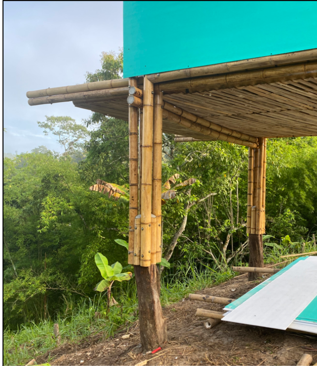
Figure B5. Finished Cantilever. Floor panels extend 1-meter past the back support beam. Notice the deflection in the beam as described in section 4.2. The ends of all exterior exposed culms (like the beam here) are enclosed with cement mortar.
