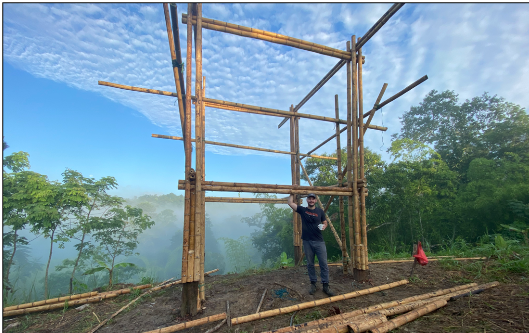
Figure B3. The author photographed with the structure towards the end of the framing process. Notice the temporary diagonal supports tied onto the right side of the frame, which also can act as an unofficial scaffolding for the maestros. The six-plus feet of vertical space under the structure allows for a secondary space to take in the views.
