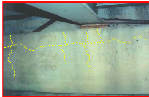
(c) Map cracking in beams
