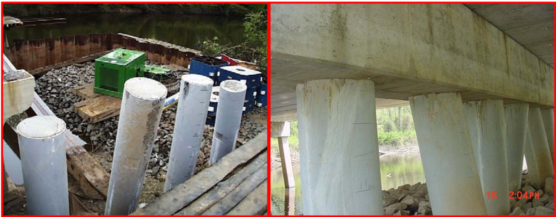
a) Photograph of composite piles installed at Pier No. 2 of the Route 40 Bridge
