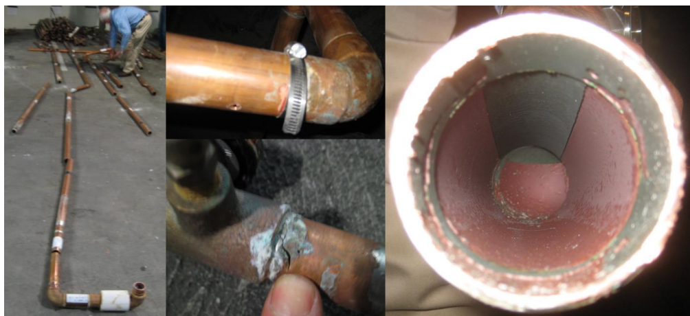
Figure 2-5. Substantial fraction of failures occurred at bends (upper center) or just downstream of valves (lower center); a very large number of failures occurred along
