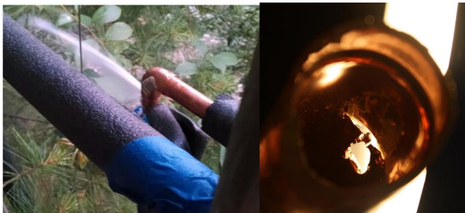
Figure 2-17. (left) Fully penetrating leak in pipe in system with small aragonite particles and (right) close-up of leak
