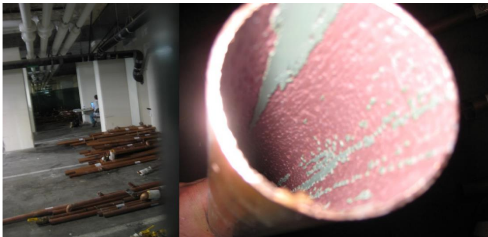
Figure 2-2. Every sample in a viewing area (left) was examined and all significant internal pipe damage was caused by characteristic erosion corrosion (right).
