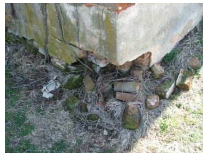
Right rear crumbling foundation
