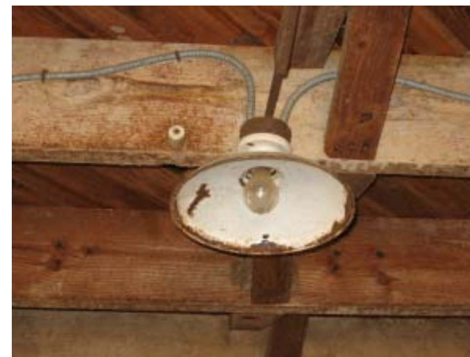
Lighting in the ceiling
