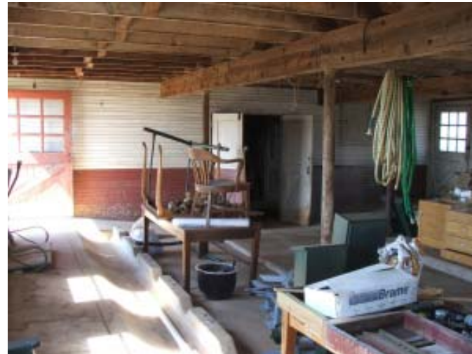
Taken from the southeastern corner looking northwest. On the far left is the feedway area, just to the right of the feedway area is the cow stall area with gutters visible. The double doors lead to mid-barn. Just to the right of the double doors is a small cabinet area that was used to hold medicines and other treatments for the animals. The door to the far right, on the northern side of the building, leads to the adjacent building (perhaps a milk storage area).
