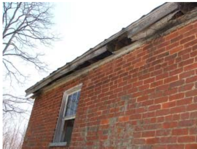
Left rear window and rotted roof
