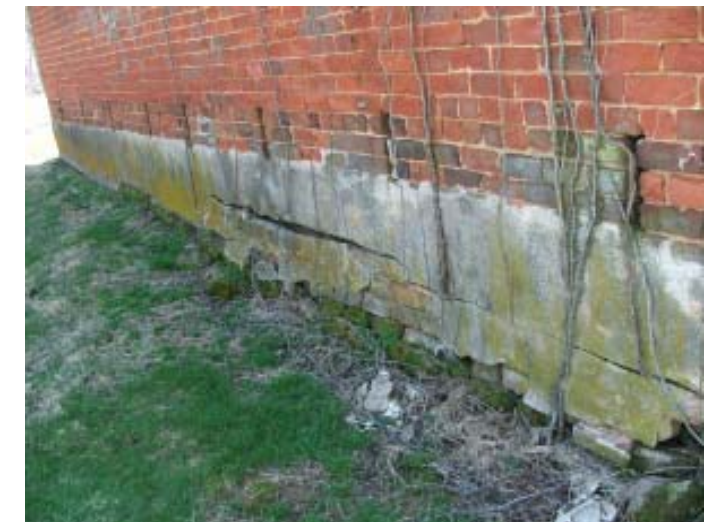
Cracked foundation at back of building
