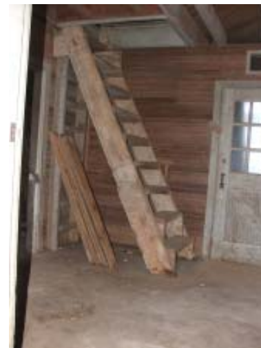
Stairs to the loft; the original ladder to the loft can be seen under the stairs.
