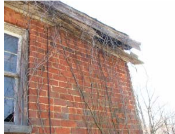
Right rear window and rotted roof
