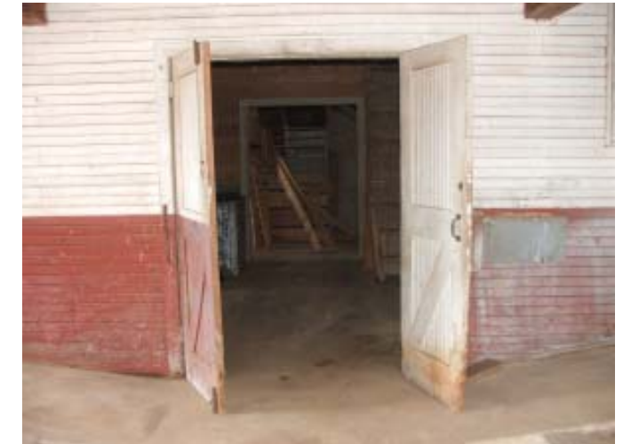
Looking from the dairy area to the stables on the western end.
