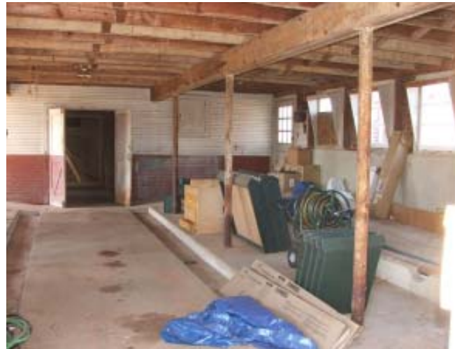
Looking west through the milking area to the center of the barn. The original gutters and the medicine cabinet are intact (to the right of the open doors).
