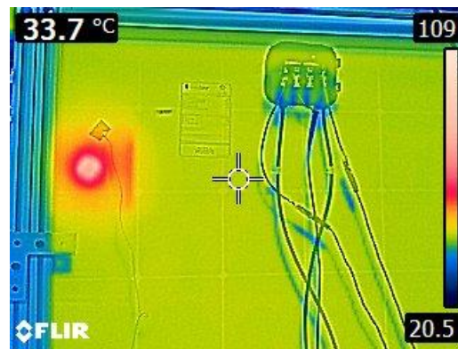
Figure 3-25 PV panel hot spot temperature measurement using a thermal imager
