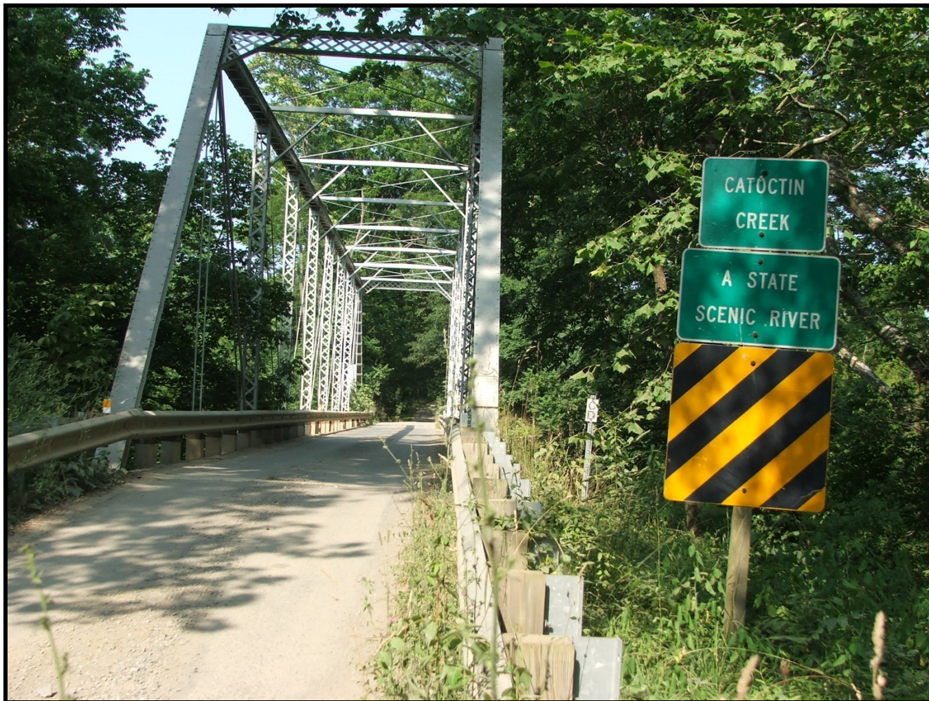
A view of the Catoclin Creek bridge on Featherbed Road in Loudoun County on June 25, 2010. Virginia's Scenic River Advisory Program is observing its 40 th anniversary in 2010.
