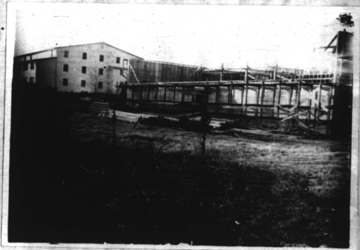
Better quality at lower cost when the apples move directly from the packing house into the cold storage (cold storage under construction).
