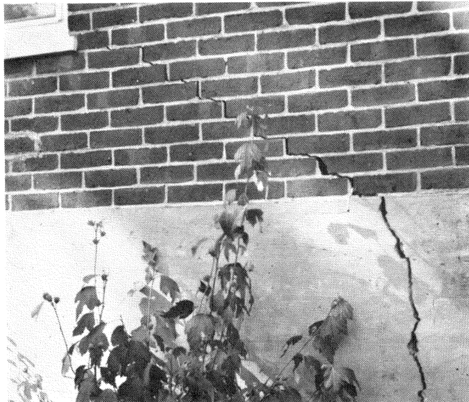
Figure 9—This foundation and wall cracked because the house foundation was not built strong enough to resist the clayey shrinking and swelling soil. A furnace in the basement was damaged and the wall had to be jacked back to close the crack and stabilize the building.
