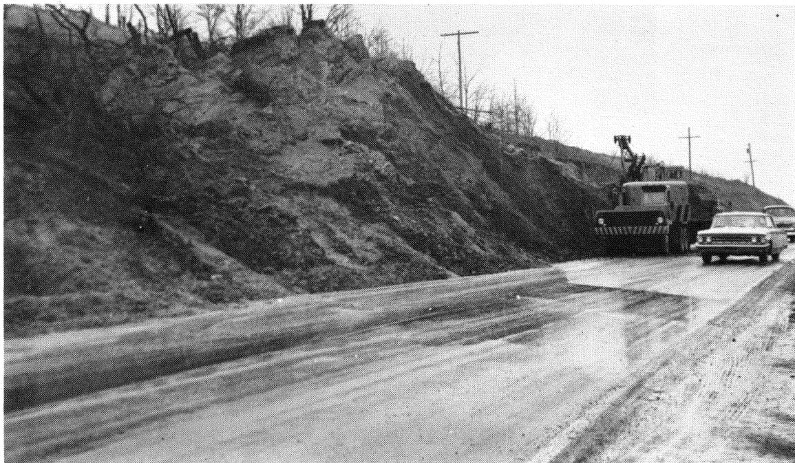
Figure 3—SLIDES CAN BE EXPENSIVE! Estimated cost of moving soil out of landslides in Southwest Virginia alone was about $300,000 in 1963.
