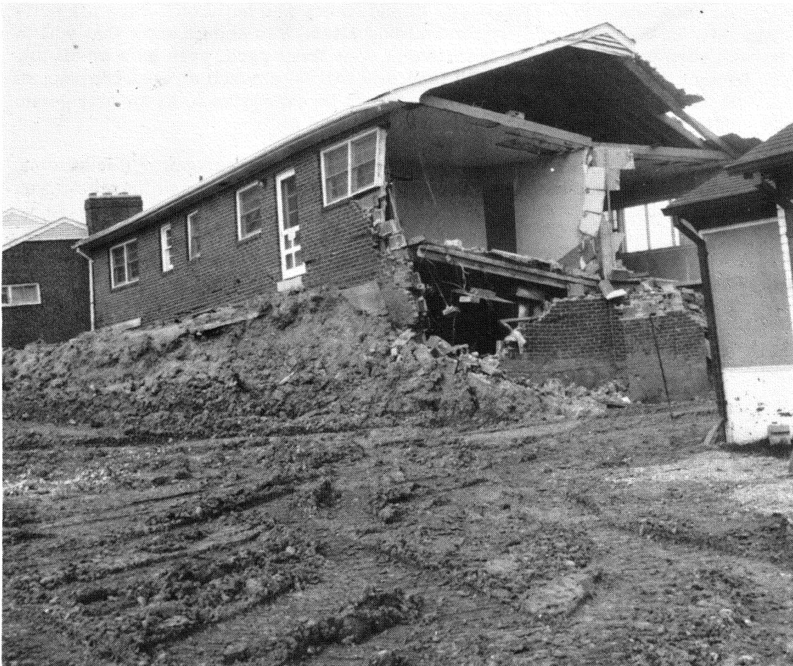
Figure 1—This is one of several new homes which were badly damaged by a large landslide in clayey sediments in the Coastal Plain of Virginia.
