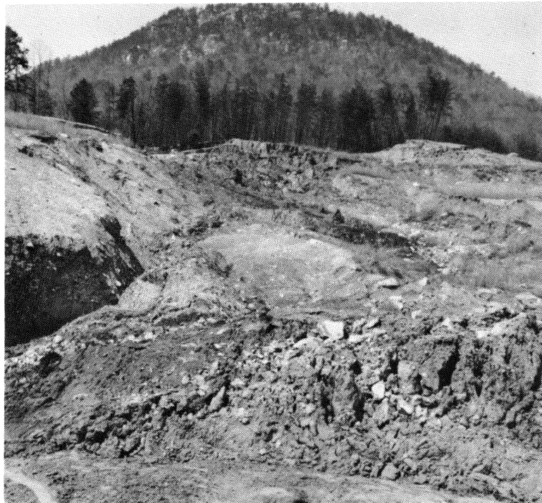
Figure 5—A LARGE LANDSLIDE IN ALLEN SOIL. NEAR HOLLINS, VA. ALONG U.S. 81. Workers have been hauling materials from this slide for many months and it is still creeping into the highway. It covers several acres and estimated cost of removal will run over $100,000.
