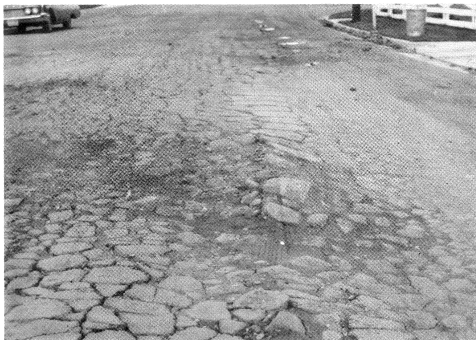
Figure 11—Soil conditions were unknown when this street was built on somewhat poorly and poorly drained clayey soils.
