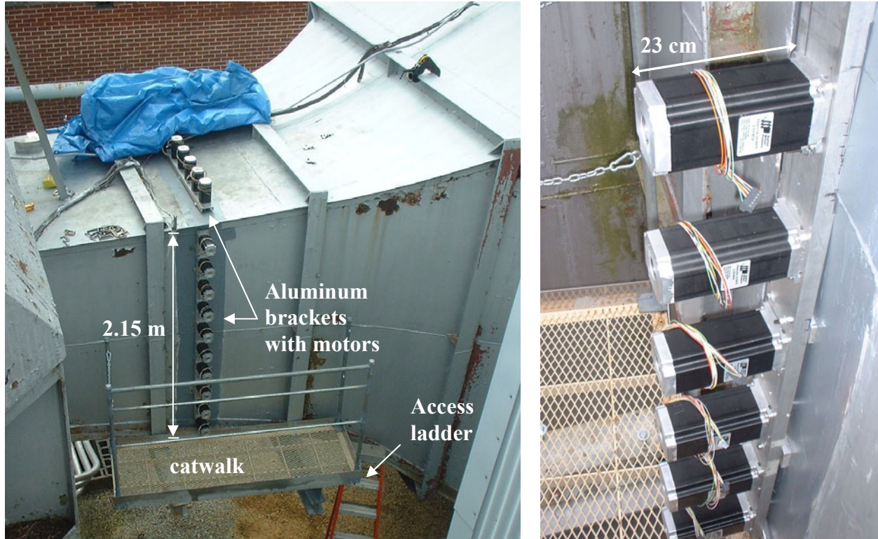
Figure 3.7. Motors and outside aluminum brackets: a) outside view of the contraction of the Stability Wind Tunnel; b) side mounted motors and bracket.
