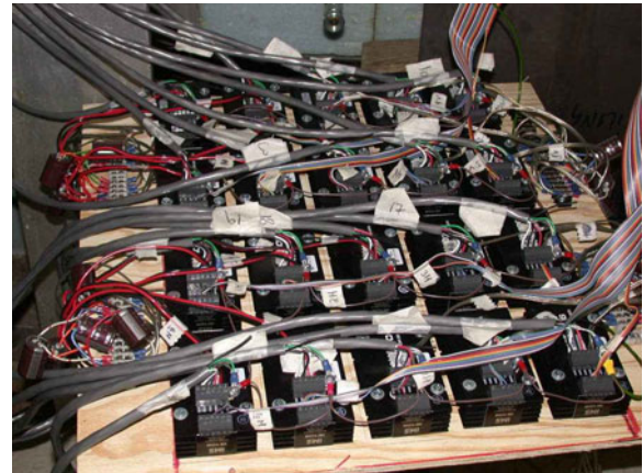
Figure 3.14. Complete array of 20 IMS IB 106 step motor drivers
