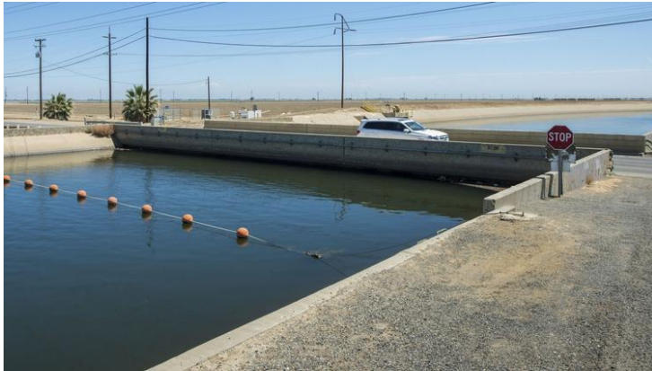
Figure 28: The Russell Avenue Bridge in Firebaugh, CA has sunk so much that it is almost touching the water in the canal it crosses (Boxall 2015)
