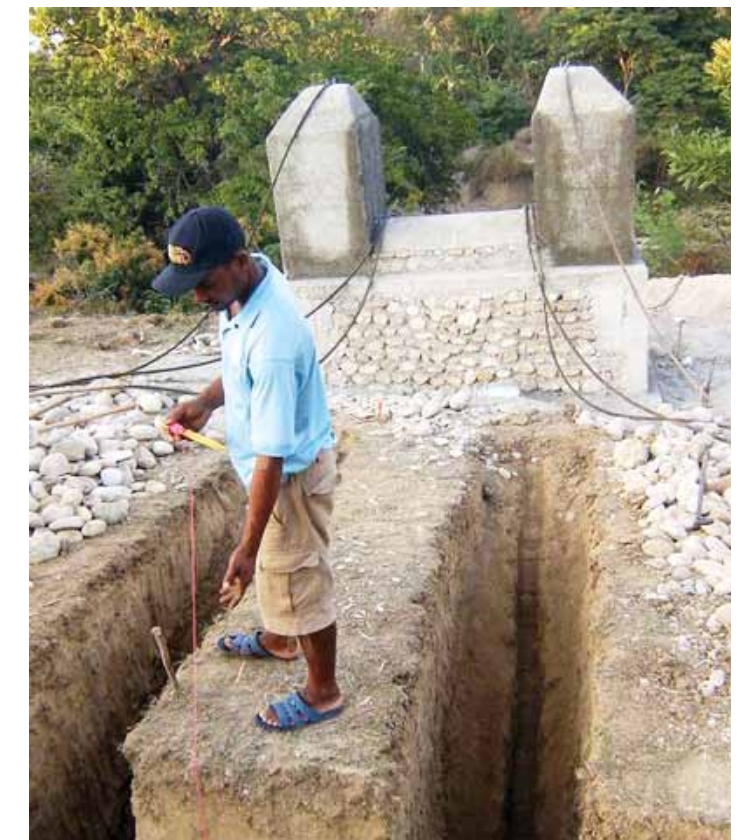
Most of the construction of the bridge was done during Bridges to Prosperity's trip to Ti Peligre over Thanksgiving break last year.
