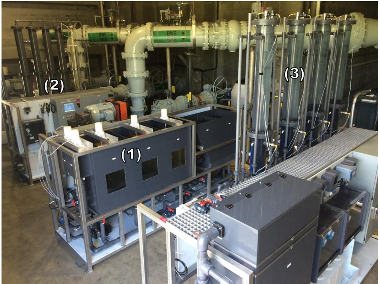
SI Figure A.2: Photograph of operational pilot plant with (1) coagulation, flocculation, and sedimentation skid, (2) ozone skid, and (3) BAC filter and GAC contactor skid.
