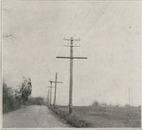
Combination telephone and 2300 volt line.
