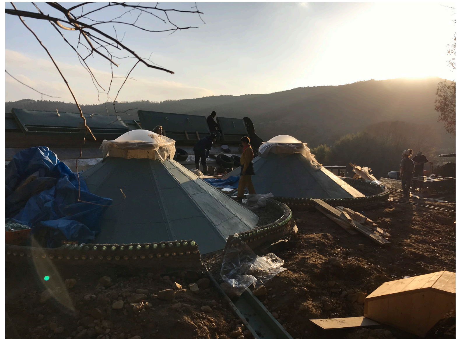
Top left and right: Photos taken on site during construction at Earthship Mima, Tokushima prefecture, Japan. 2018
