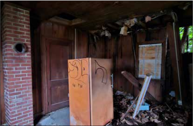
S6: View showing the chimney and some of the damage caused by overgrown vegetation in the second office.
