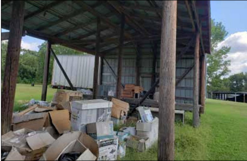
L5: A variety of trash and debris sits beneath this structure.
