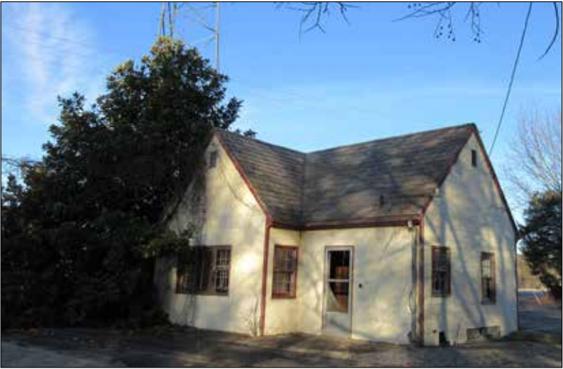
S3: View of the building exterior looking northwest. Vegetation is starting to overtake one portion of the structure.
