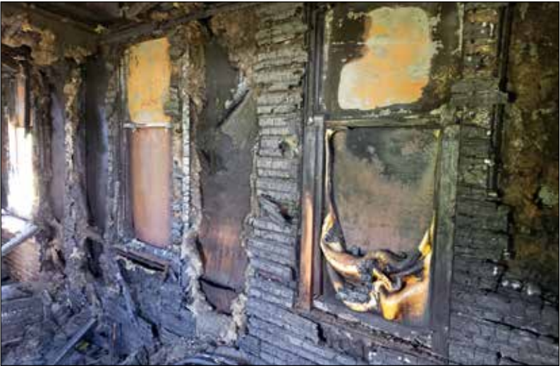
C6: The caboose sustained significant damage during the fire, which revealed frames to several additional windows that were previously covered up.
