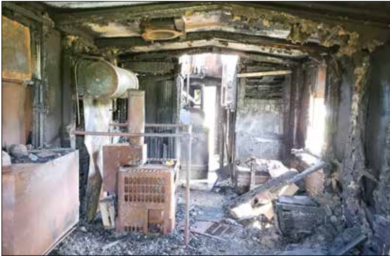
C5: The caboose interior was badly damaged by arson last year.
