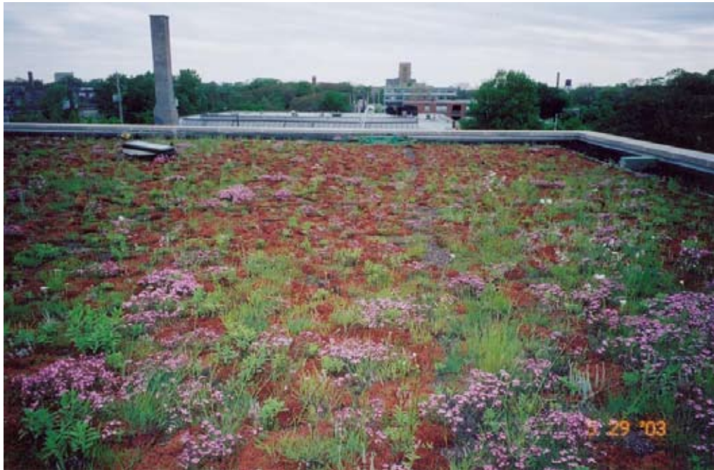
Green Roof, Center for Neighborhood Technology, Chicago, Illinois
