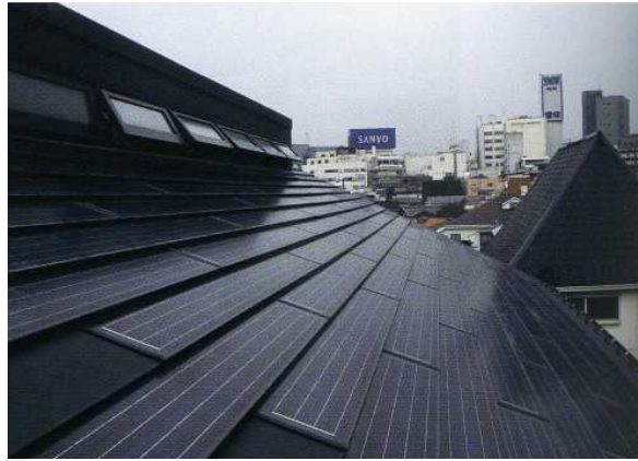
Fig 2.7 – Rooftop PV array 11
