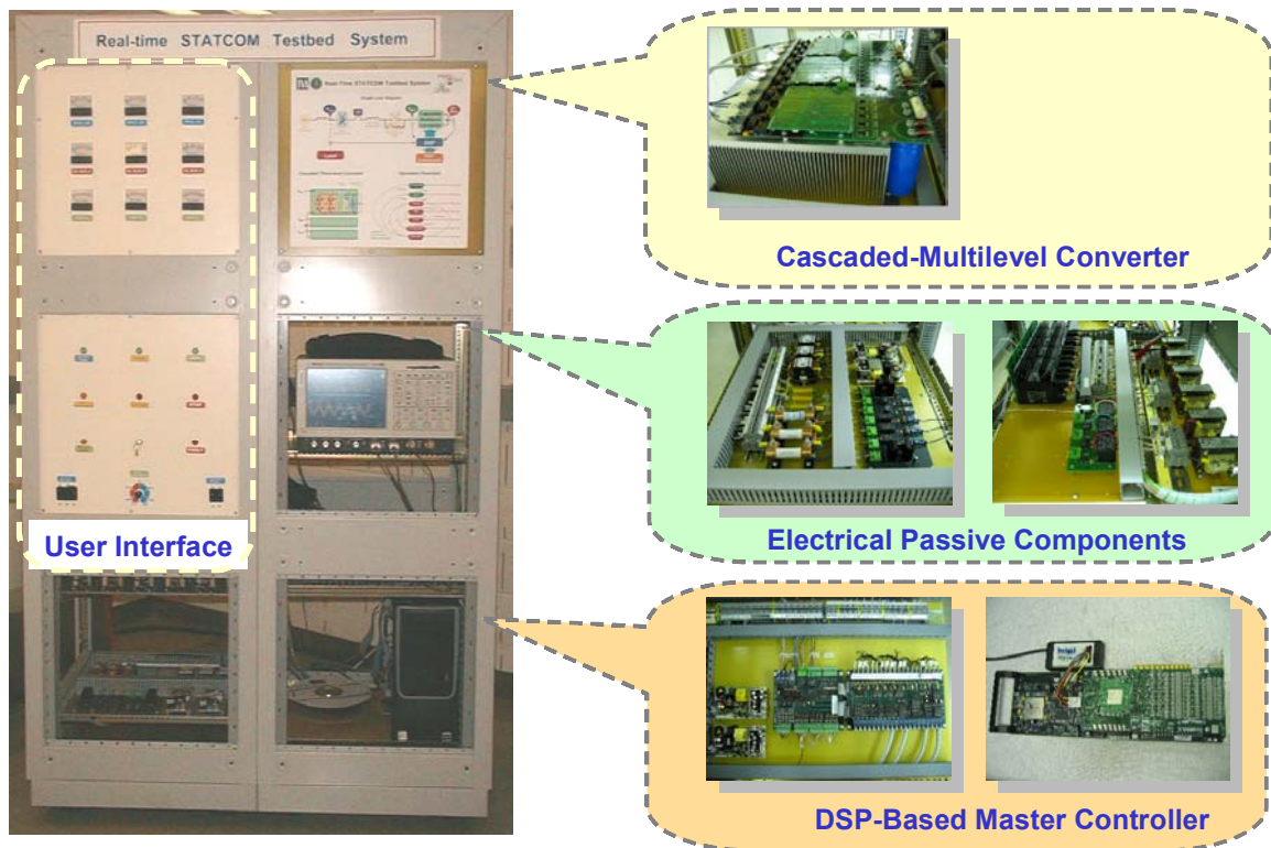
Figure B - 4. Pictures of the IGBT-CMC-based STATCOM hardware prototype and its components.
