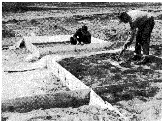
Construction of an experimental golf green, consisting of 12 modified soils, for evaluation of soil compaction, aeration, and water requirements.
