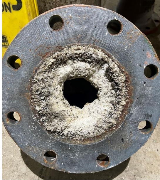
Figure 3: Scale within a removed pipe bend at HRSD's Atlantic Treatment Plant transporting digestate to the final dewatering centrifuges.
