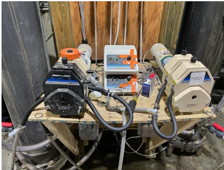
Figure 63: Pilot feed flow setups - the first continuous feed iteration with 3/8th-inch tubing and T-fittings.
