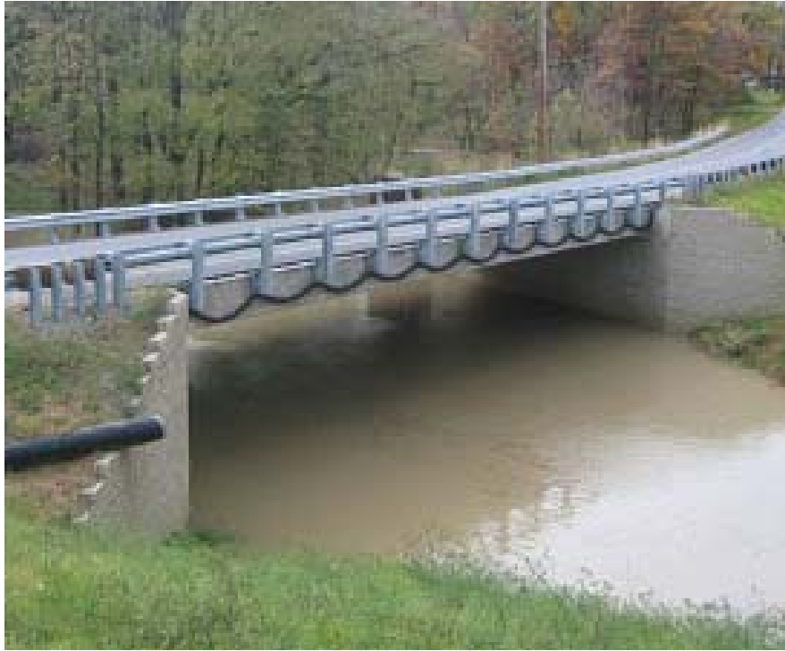
Figure 10: Bowman Road Bridge FHWA (2011). "Geosynthetic Reinforced Soil Integrated Bridge System (GRS-IBS)." Every Day Counts Presentation , U.S. Department of Transportation. Used under fair use, 2014.
