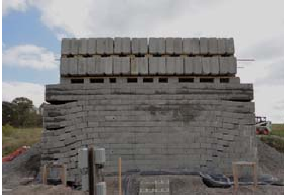
Figure 30: Virginia Tech Abutment Wall after Testing Kost, A., Filz, G., and Cousins, T. (2014). "Differential Settlement of a GRS Abutment: Full-Scale Investigation." Virginia Center for Transportation Innovation and Research Charlottesville, VA. Used under fair use, 2014.
