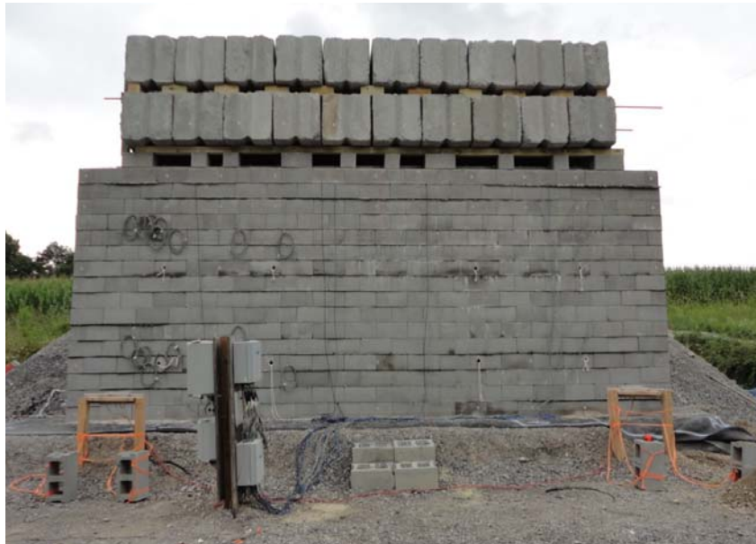
Figure 28: Photograph of the Virginia Tech Abutment Wall Kost, A., Filz, G., and Cousins, T. (2014). "Differential Settlement of a GRS Abutment: Full-Scale Investigation." Virginia Center for Transportation Innovation and Research Charlottesville, VA. Used under fair use, 2014.
