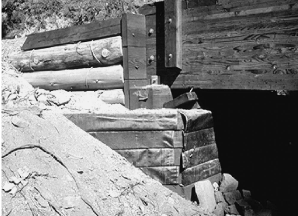
Figure 5: Feather Falls Trail Abutment without Facing Keller, G. R., and Devin, S. C. (2003). "Geosynthetic-Reinforced Soil Bridge Abutments." Transportation Research Board, Washington, D.C. Used under fair use, 2014.
