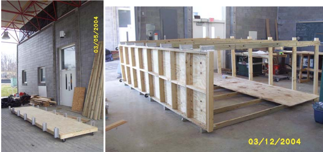
Figure 3.15: Wood studs are bolted to stand-vertically by being sandwiched with pairs of angled steel plates
