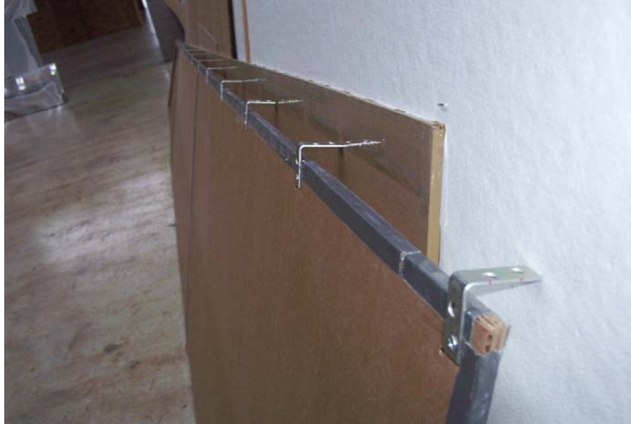
Figure 3.26: Brackets are screw fixed at a foot apart along the length of the piece of enclosure
