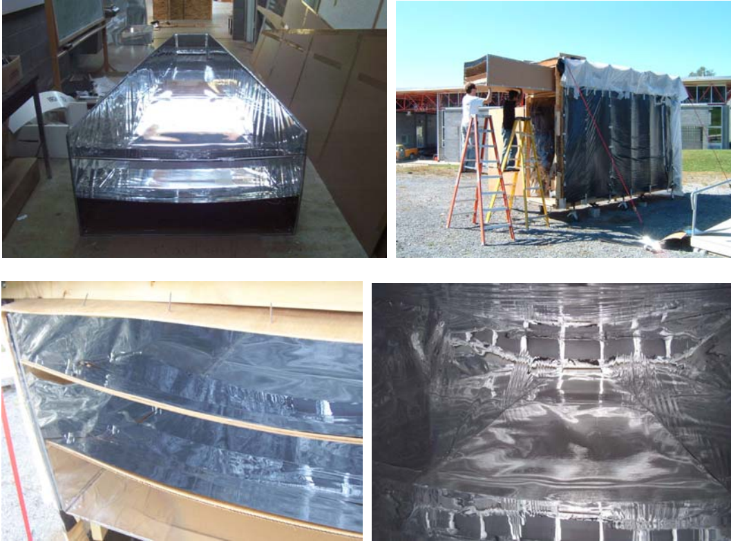
Figure 3.28: The installing of the finished tapered geometric mockup into the ceiling cavity of the test cell
