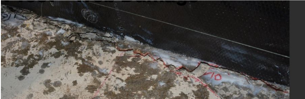
Figure 4.47: Final Condition S2FL Base Crack
