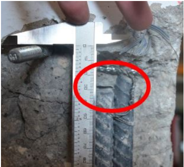
(b) Lap Splice Slip Uncovered
