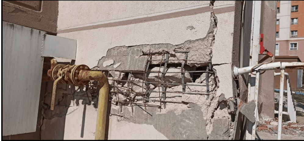
(a) Web Wall Crushing, Bar Buckling, Out of Plane Failure. Turkey 2023 (Işık et al., 2024)
