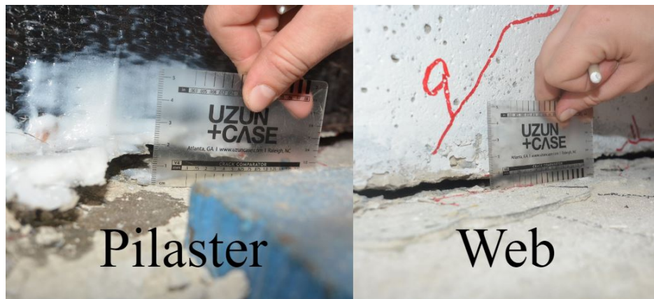
Figure 4.31: Final Base Crack of Specimen S1FP
