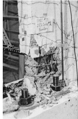
(b) Toe Concrete Crushing and Bar Buckling (Thomsen and Wallace, 1995)
