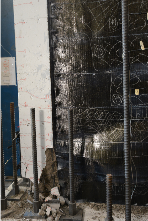
Figure 4.21: South Toe and FRP Delamination Photo of Specimen S1FW - Final Damage State
