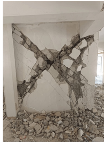
(c) Diagonal Tension (shear) Damage. Turkey 2023 (Işık et al., 2024)
