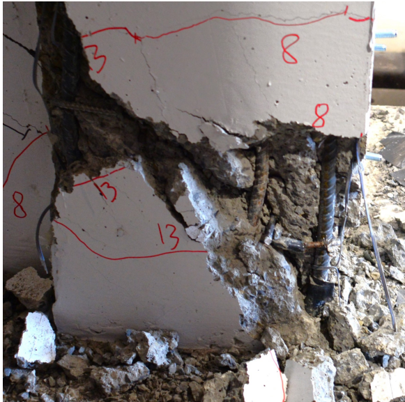
Figure 4.8: S1 Crushed Toe Close Up
