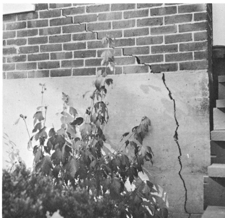
Plate 14. Improper footings in swelling and shrinking clayey subsoils, such as Carbo, Lodi, Frederick, and Groseclose soils, may cause cracked walls and basements.
