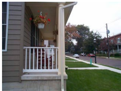
Porch depth insufficient
