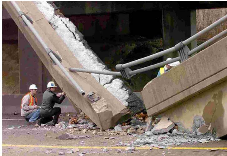
Figure 11: Collapsed Fascia Beam of the Lake View Drive Bridge (Harries 2009)
