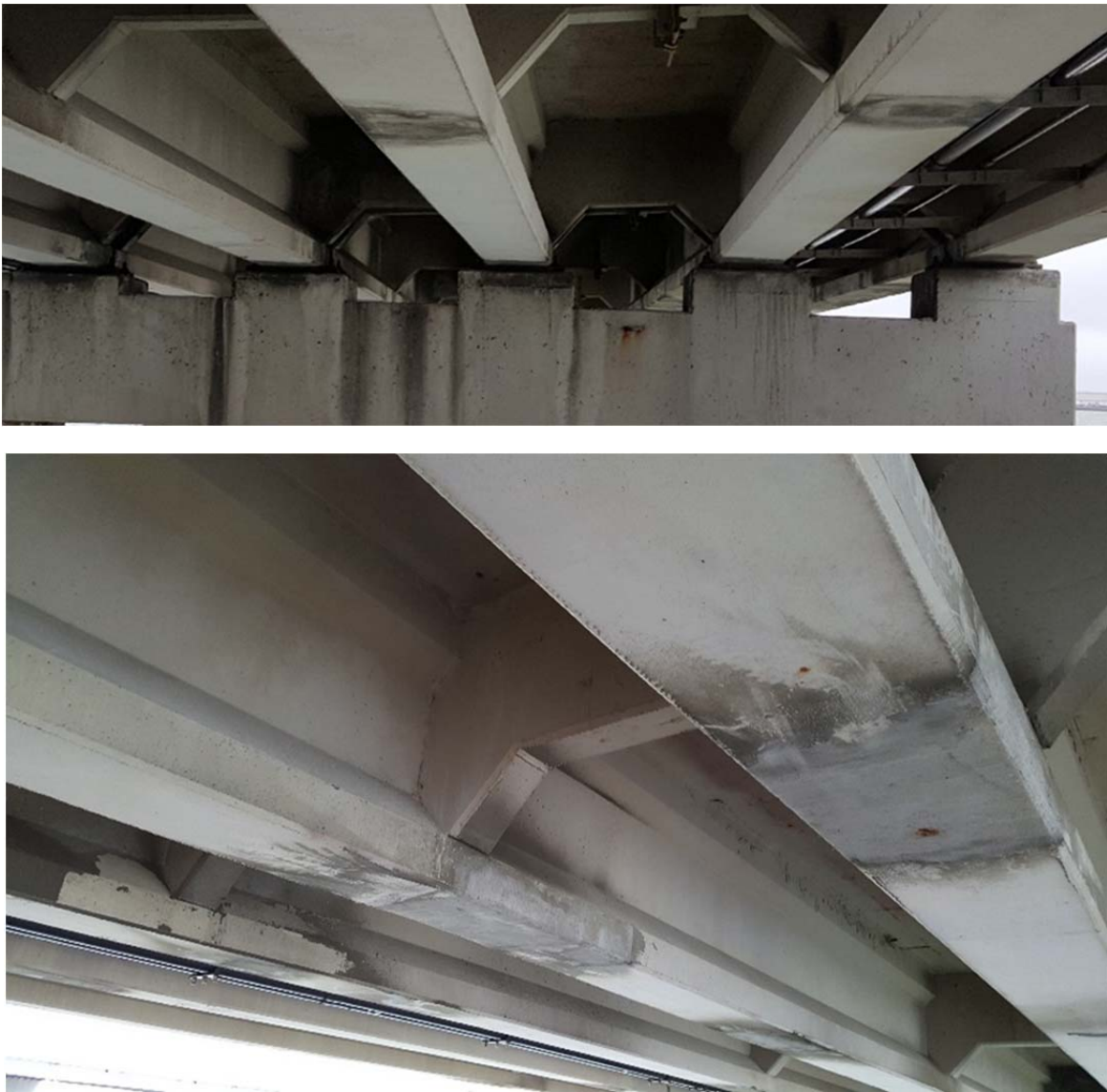
Figure 26: Patching on Girder Bottom Flanges
