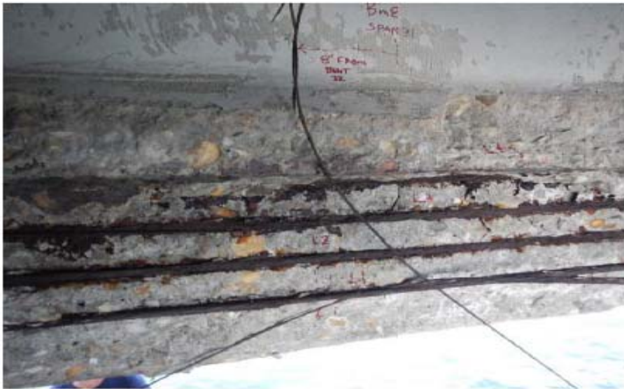
PHOTO J (BEAM 8, SPAN 31)
