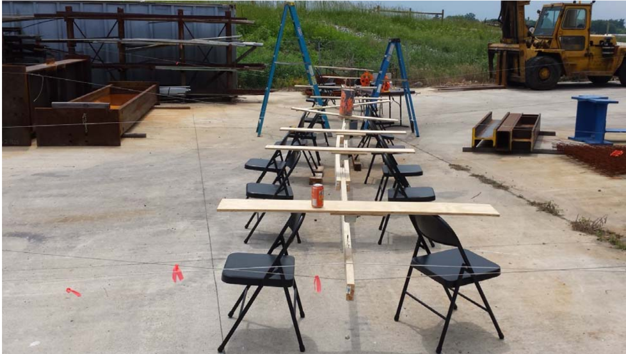
Figure 35: Mock Setup of the Cable Suspended System
