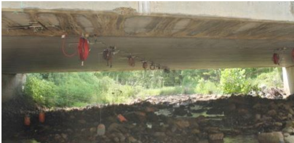
Figure 50. Overview of instrumentation
