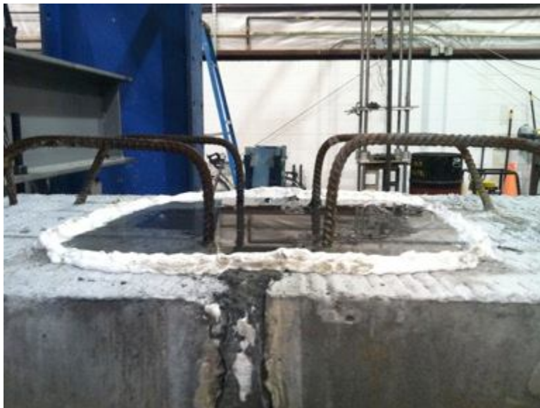
Figure 37. Water ponding for voided slab
