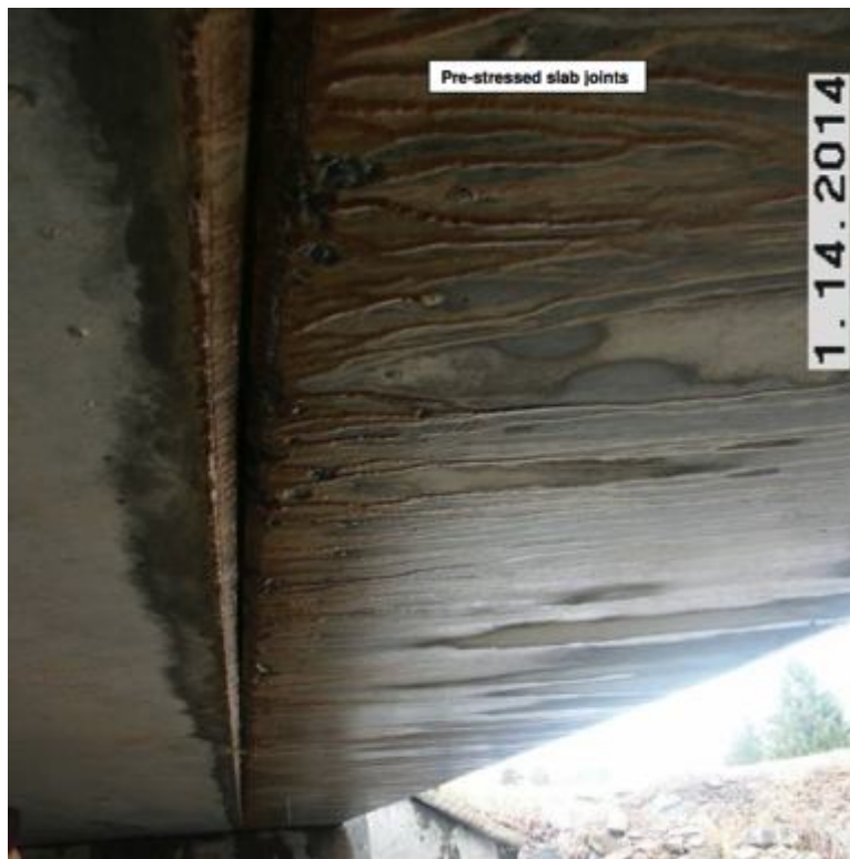
Figure 38. VDOT visual inspection report picture of downstream joint leaking
