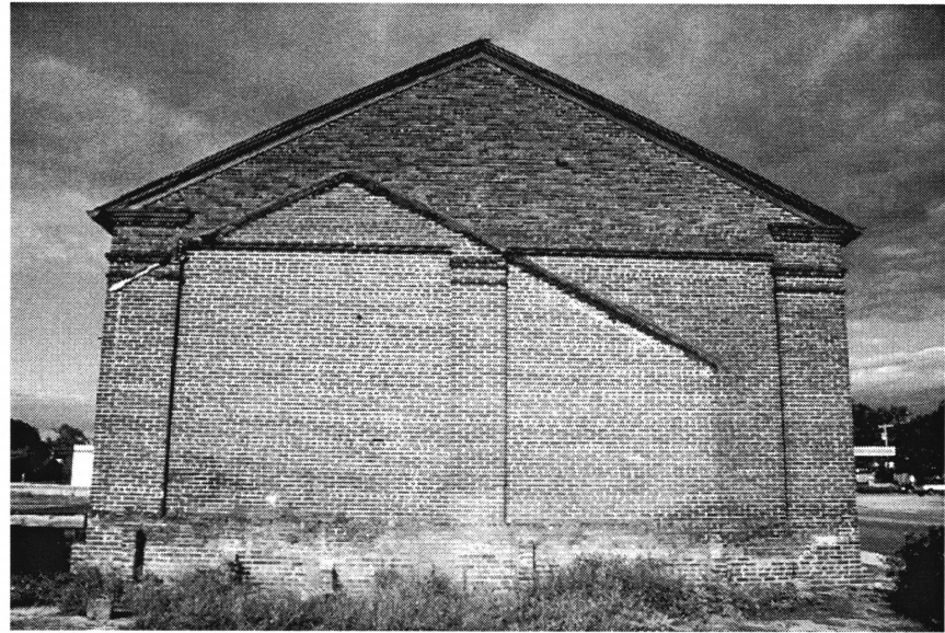
FREIGHT WAREHOUSE, TARBORO: 1994 SCAR LEFT BY REMOVAL OF ADDITION
