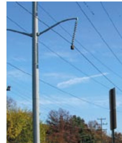
Utility corridor located in front of Barcroft Rec Center along Four Mile Run Drive.
