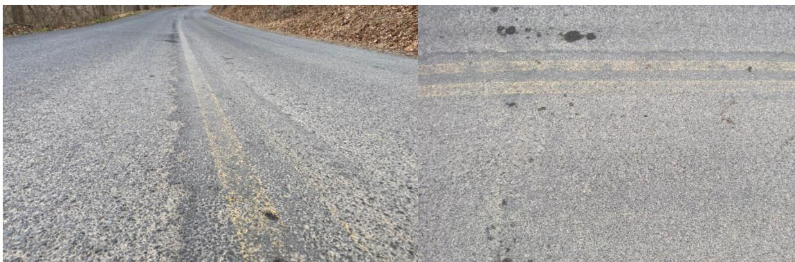
Figure 22. Irregularities/Rutting along the route
