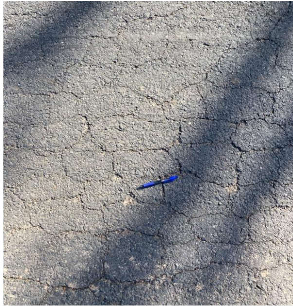
Figure 19. Fatigue cracking in the center of the road
