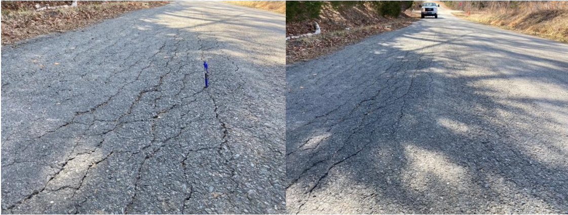
Figure 18. Fatigue cracking at the edge of the road
