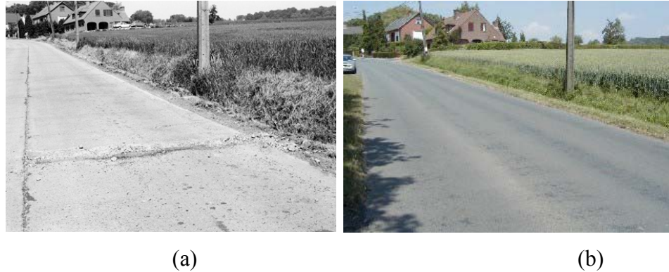
Figure A-2. Comparison between a Road in Belgium: Before Repair and Eleven Years After Repair (after Al-Qadi et al. 2002)
