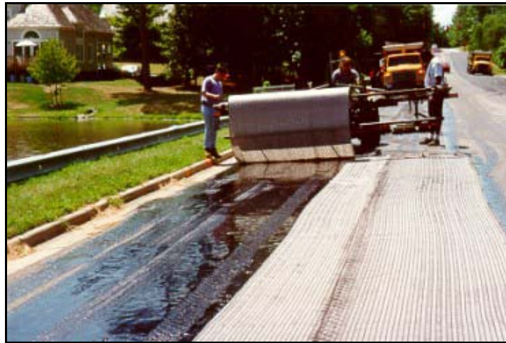
Figure A-3. Unrolling Process of a Geotextile after Application of a Tack Coat
